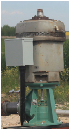
Photo A: Regenerating pump and line shaft turbine
